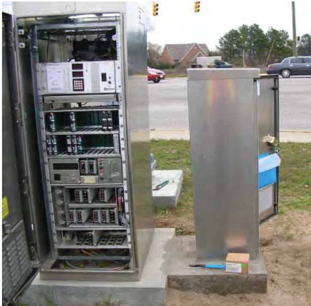
Battery Back-up System (cabinet adjacent to signal cabinet)
