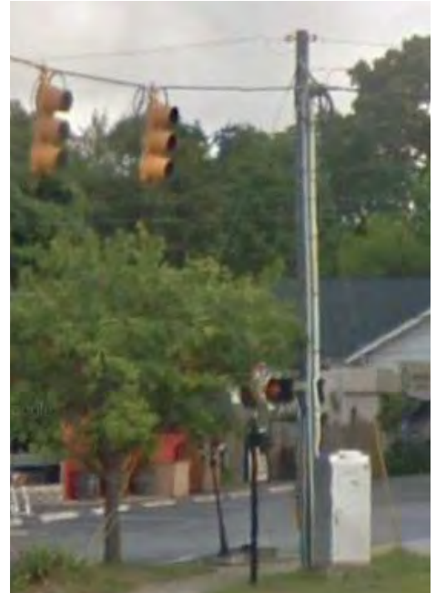
Wood pole with Cabinet
