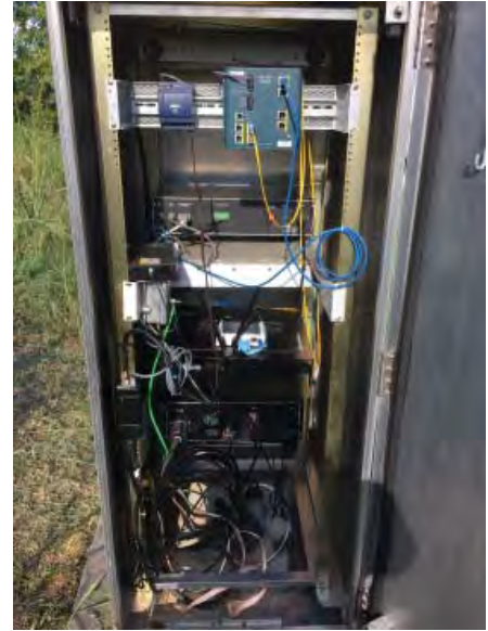
Switches in Cabinet
