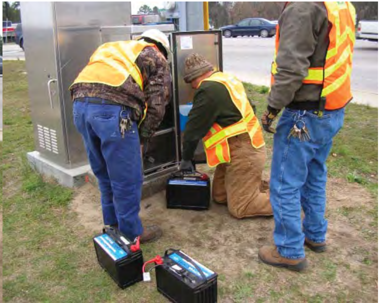
Battery Back-up System (batteries)
