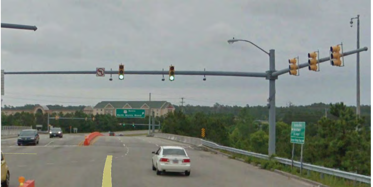
Dual Mast Arm, Galvanized, Non- decorative, with luminaire Standard yellow pedestrian heads and signal heads
