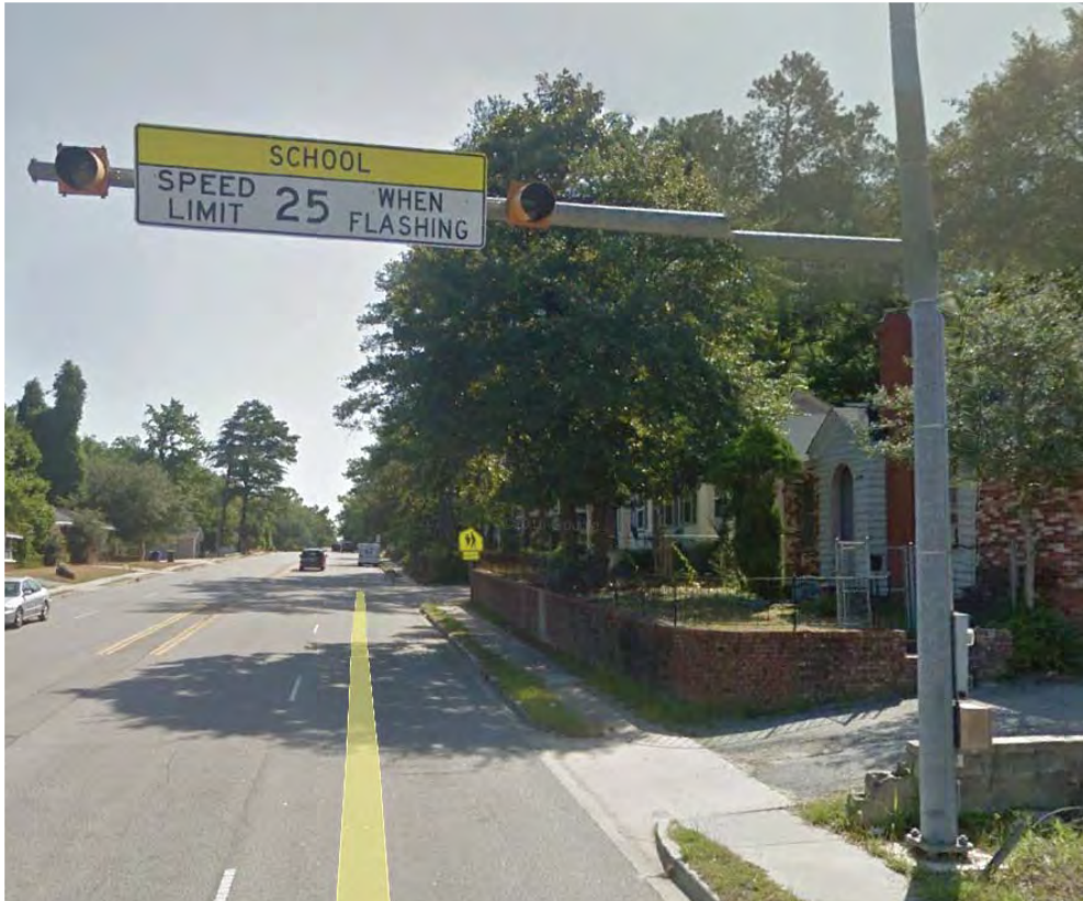
Flasher Cabinet at School Zone
