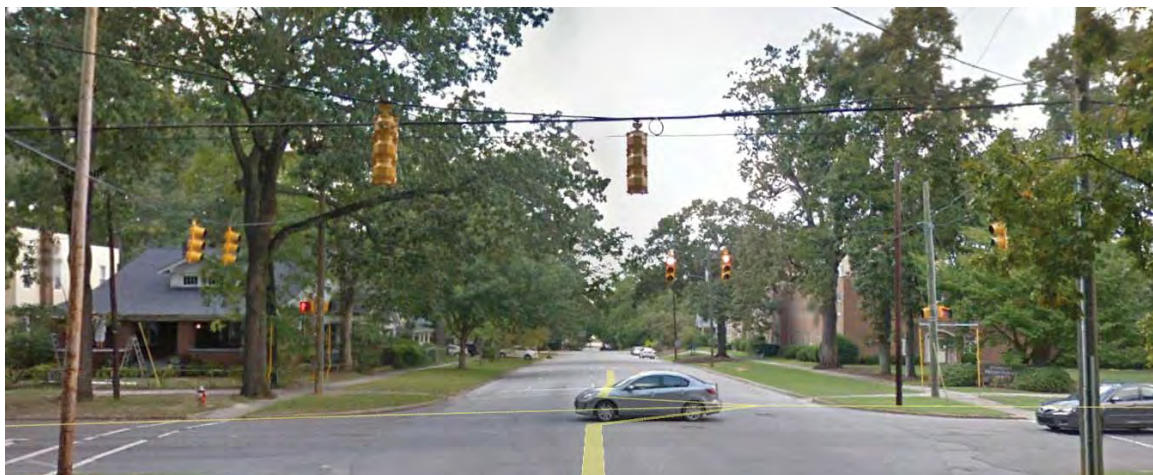
Signal with wood poles
