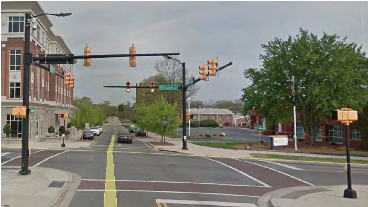
Dual Mast Arm, Powder coated, Non- decorative, with luminaire mast arm Powder-coated pedestrian pole, standard yellow pedestrian heads and signal heads
