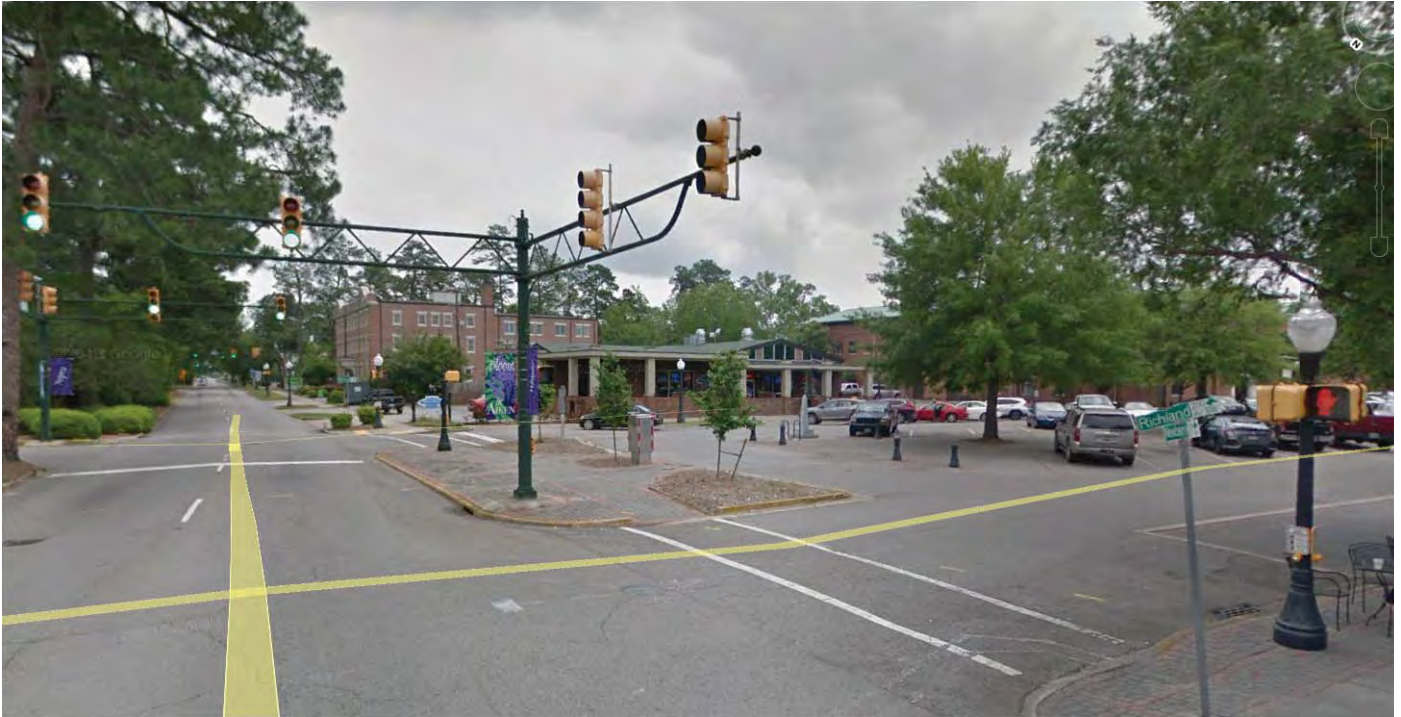
Dual Mast Arm, Powder-coated, Decorative (skirt, truss style arm), no luminaire Standard Yellow pedestrian heads and signal heads Decorative/Powder-coated pedestrian poles with luminaires (for street lighting)
